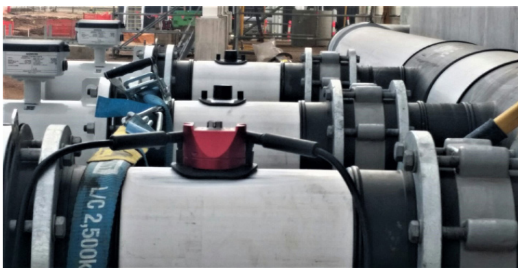
More than eighty sensor points were to be joined to pipes ranging in size from 225mm to 630mm. Due to the compact nature, several sensors were often designed to be installed circumferentially around the pipe.
